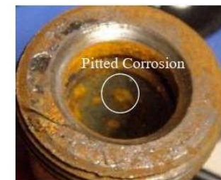
Figure 2.4: Pitted Anoxic Corrosion
